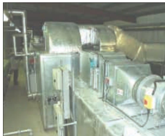
Typical cleanroom air movement system
